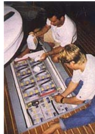
This installation of wet-cell batteries has separate cranking batteries side by side.
